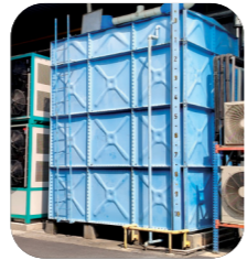
Photo of rainwater harvesting system at QL Kitchen Sdn. Bhd.
