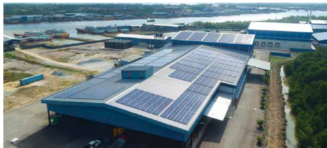
Solar panels installed on the roof of our plant at Endau, Johor.
