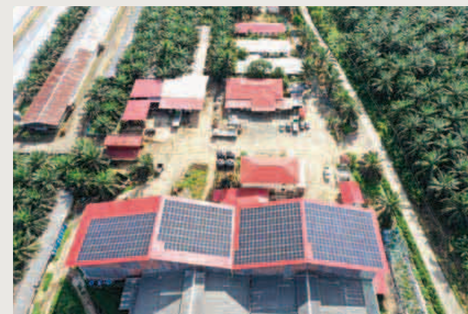
New solar panel installed at organic fertiliser plant, Tawau
