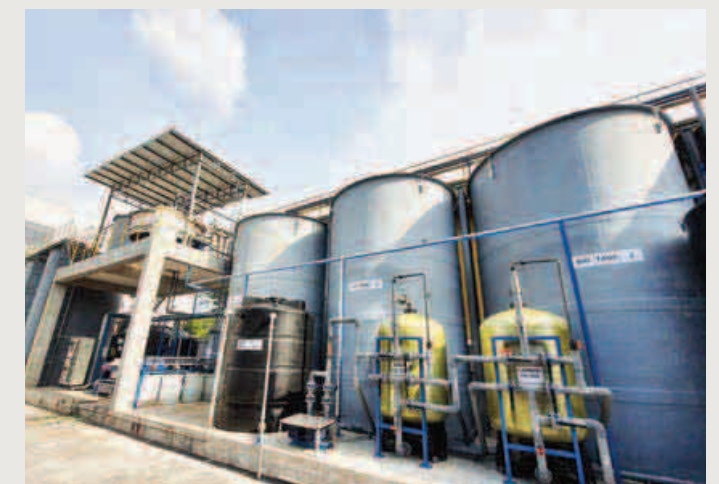
Water Treatment installation at client's facility
