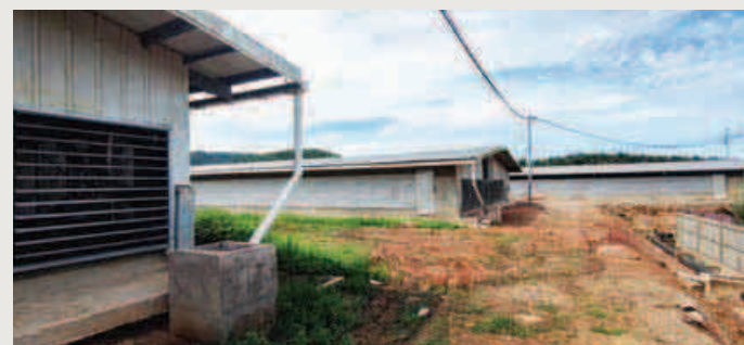
Rainwater harvesting system in QL Breeder
